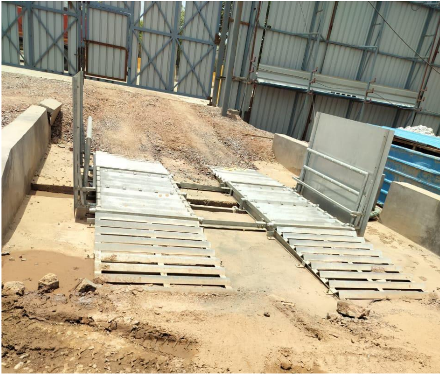
Figure 1 Wheel washing facility at site
